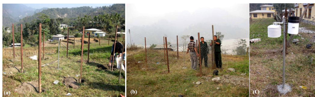
Fig. 2 Establishment of Meteorology station (a) iron post erecting, (b) mesh wire fencing around iron post and (c) installed HOBO loggers (Rain gauge and Temperature, Humidity)
